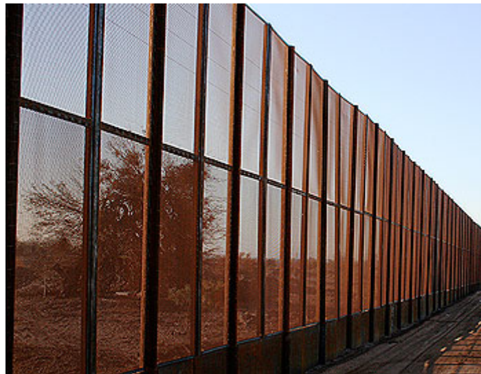
Figure 13. Metal mesh fence in Yuma Sector 245
