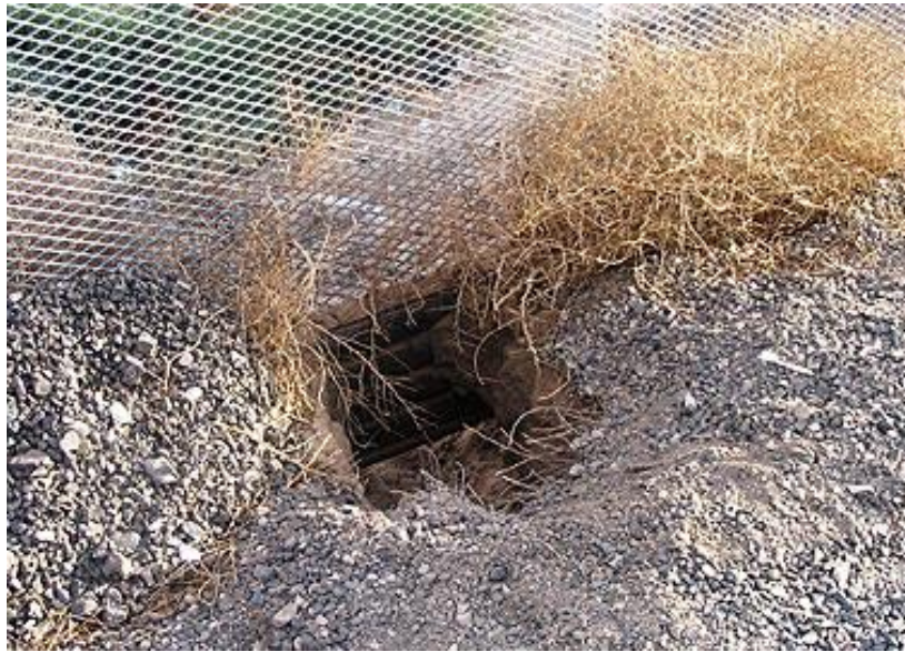
Figure 14. Fence breach in Tucson 246
