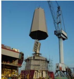
Figure 3. Integrated mast structure for the US LPD-17 amphibious land platform. Image extracted from [12]. The image shown is only for illustrative purposes.
