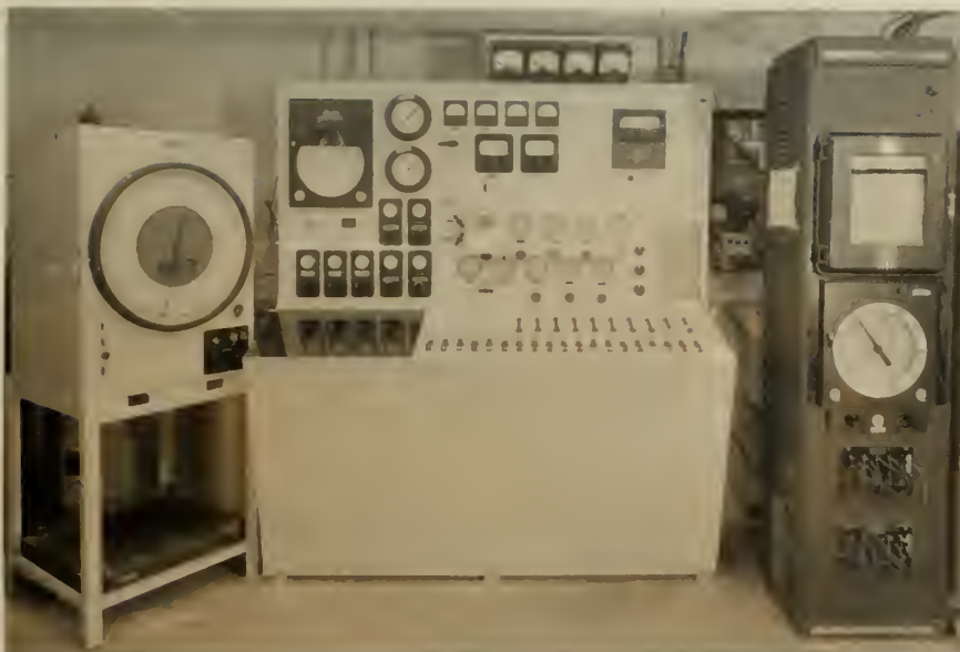
Compressor Plant Motor and Valve Controls Reservoir Pressure and Temperature Regulators Plant Pressure and Temperature Indicators
