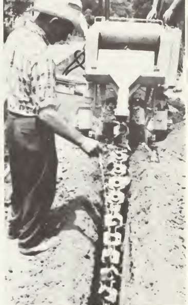
● A construction company worker measures the depth of the trench which will be used for distribution pipeline in Rosiclare.
