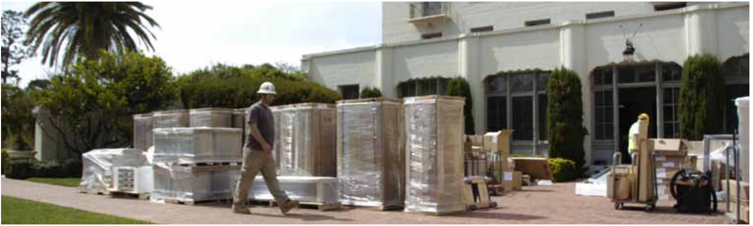
Construction crews work on the Herrmann Hall first floor renovation project. (U.S. Navy photo by MC1 Leonardo Carillo)
