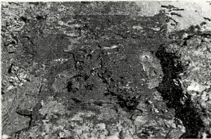
Figure 31. Photo from area of severe erosion showing evidence of pholad burrowing.
