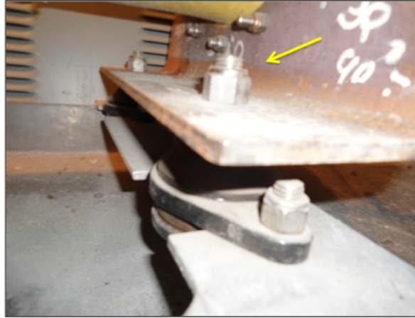
Figure 69: Vibration Mounts for Ventilation Fan on SENECA.
