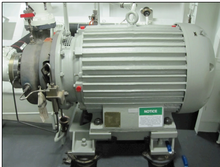
Figure 34: Robust Vibration Mounts on Fire Pump #1 on USS MICHAEL MURPHY.
