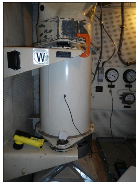
Figure 37: Forward Ventilation Fan Under the Bridge on the USCGC SENECA.
