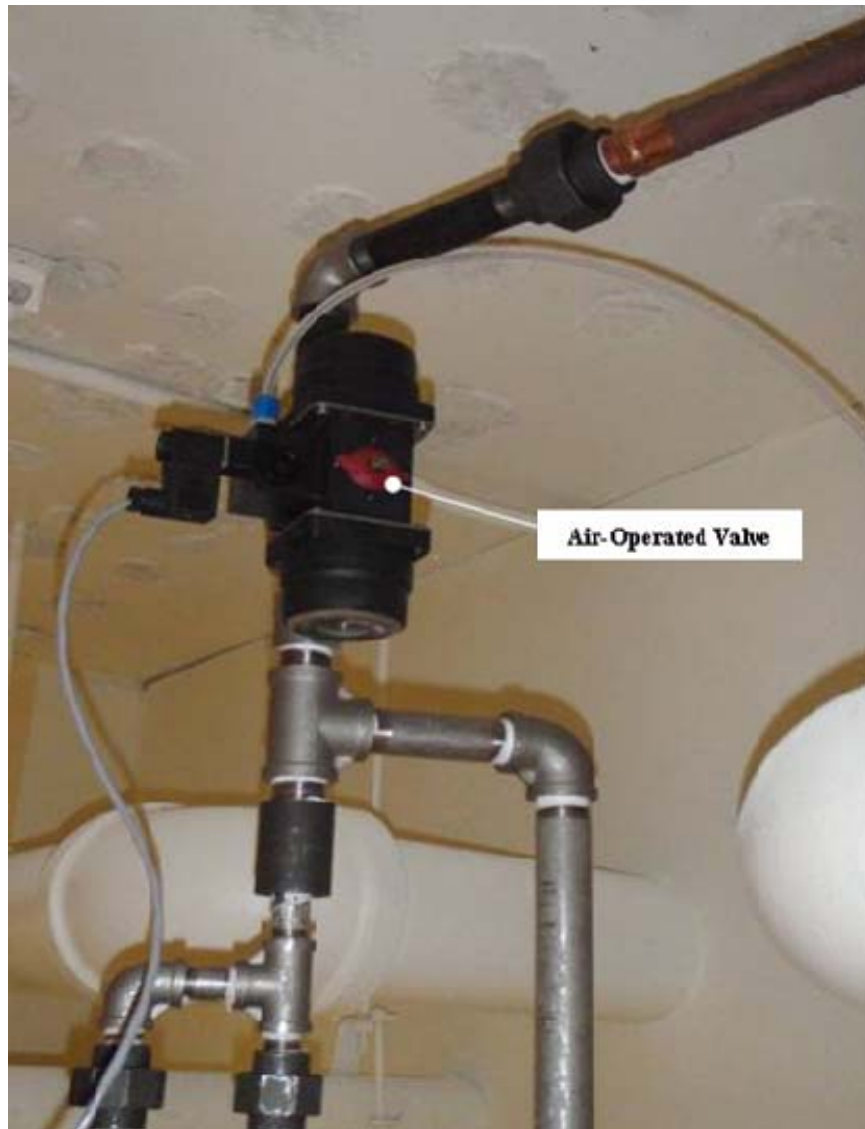
Figure 14. Exhaust System's Pneumatic Ball Valve
