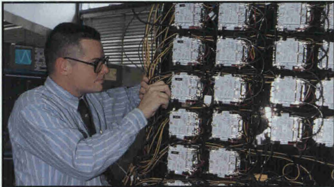
Marine Capt. Tom Langolis works on one of the magnetic switches in the simulated Surface Combatant 21 power distribution system.
