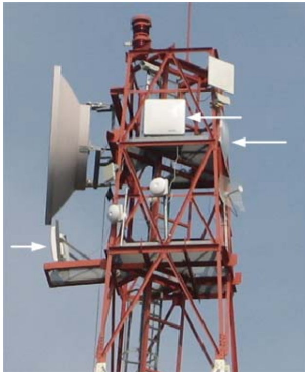
Figure 11. Phased array antennas mounted on Comms Tower on Ao Manao Airbase in Thailand.
