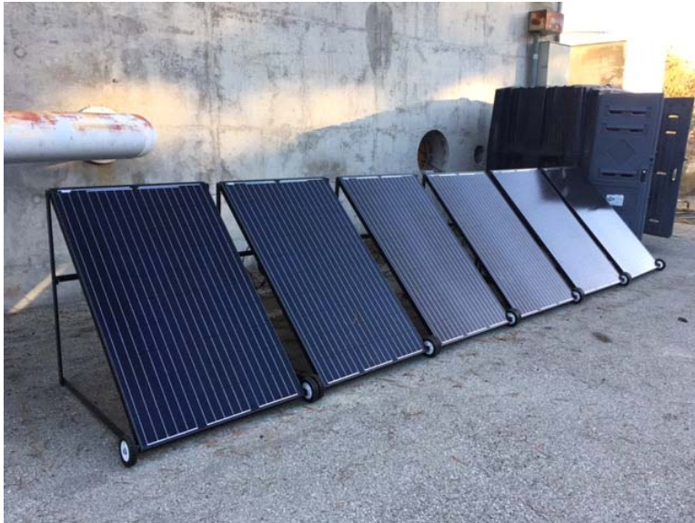
Figure 4. Array of Solar Panels.
