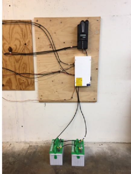
Figure 8. Batteries, Breaker Panel and Charge Controller Wiring Configuration.
