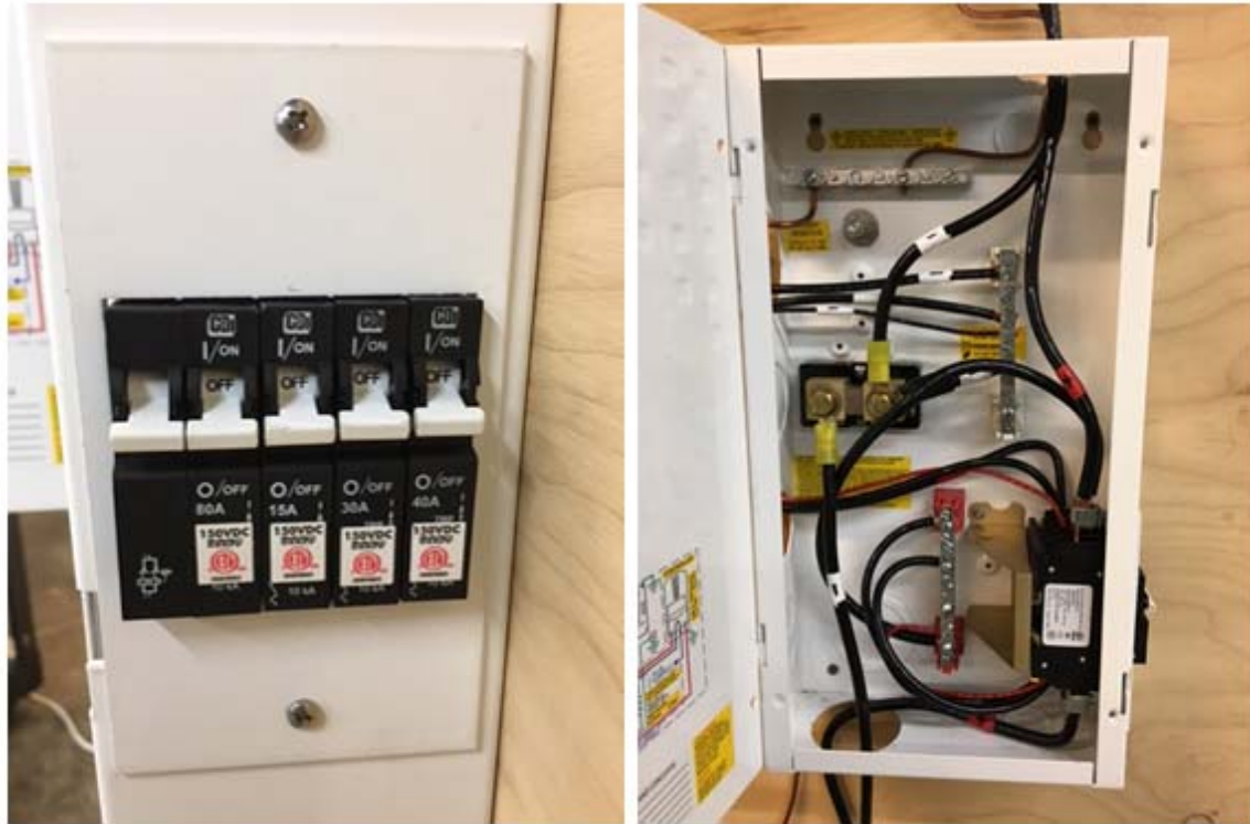
Figure 7. Breaker Panel Wiring Configurations.
