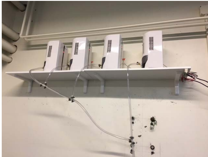
Figure 10. Dehumidification Units Configuration.
