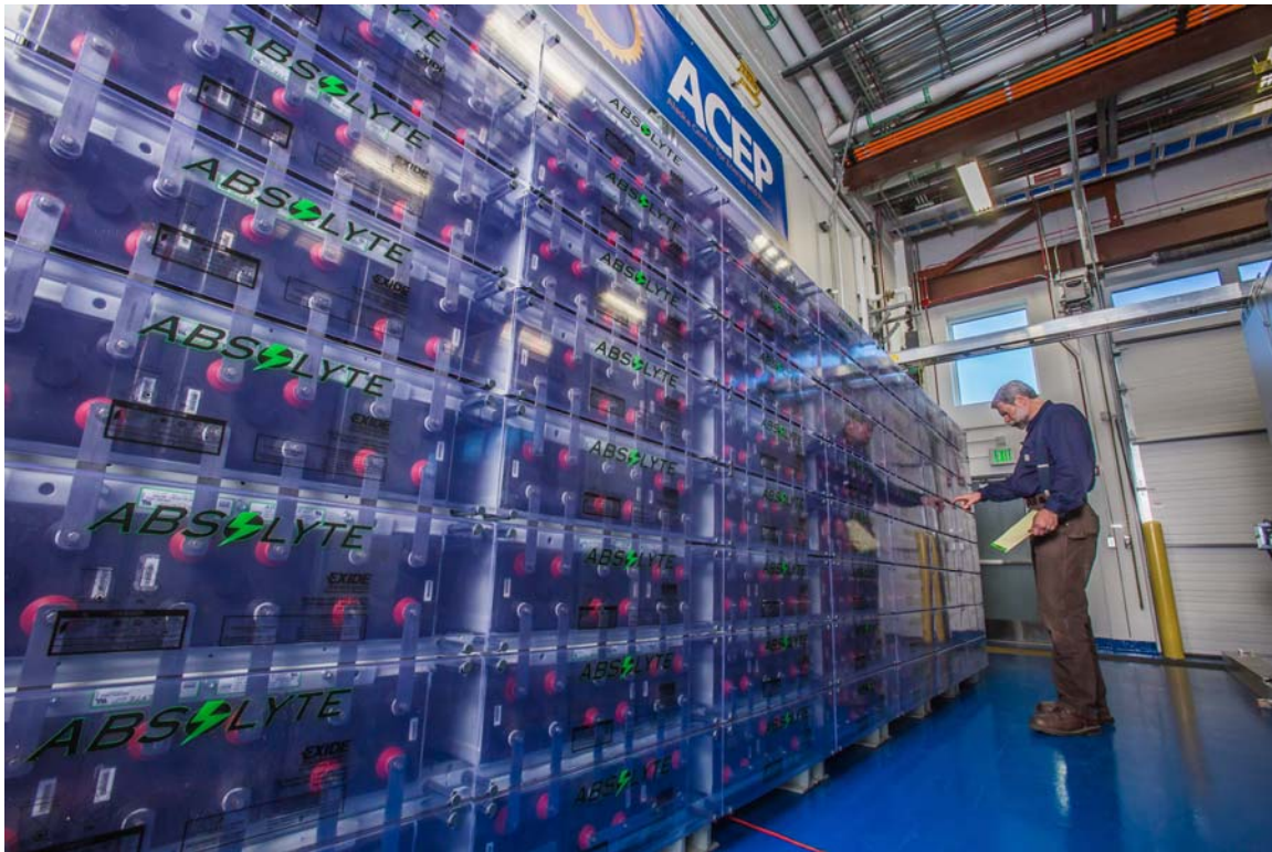
Figure 7 Secondary Battery Bank at Alaska Center for Energy and Power. Source: [26].
