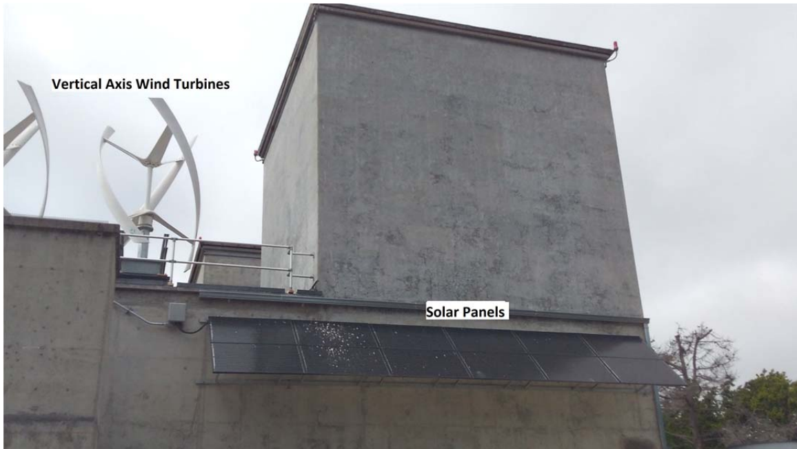
Figure 13 Solar Panel Array and Vertical Axis Wind Turbine at NPS IMPEL
