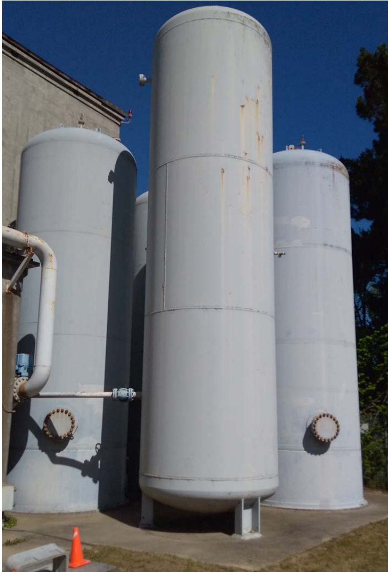
Figure 14 Four Large Compressed Air Storage Tanks at NPS IMPEL
