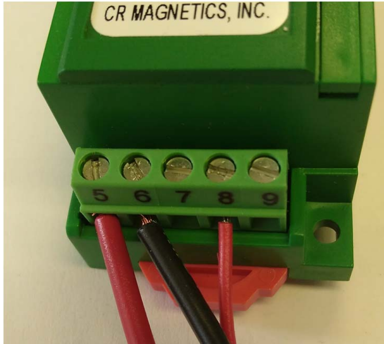
Figure 36 Voltage Transducer Output and Power Source Terminal
