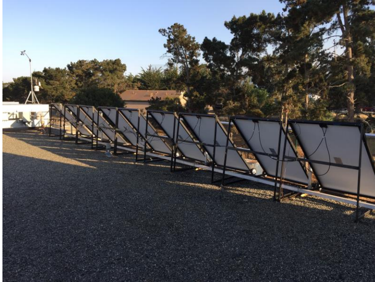
Figure 9. Picture of Solar Panels on the Roof
