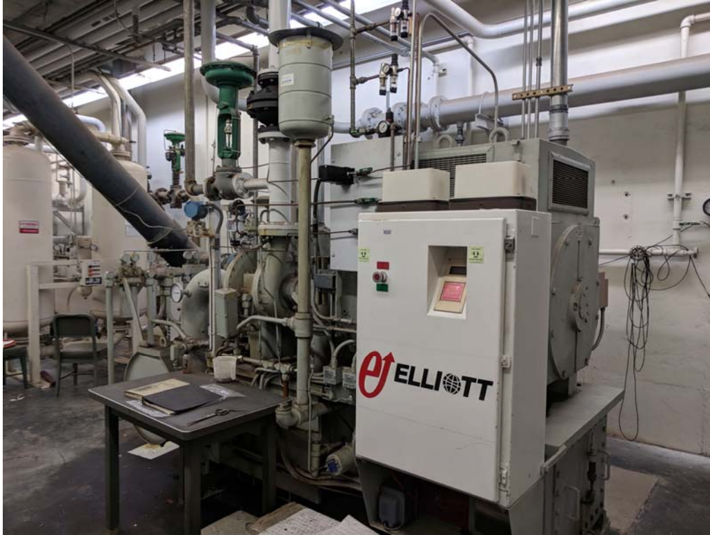
Figure 6. 500 kW Elliot Compressor
