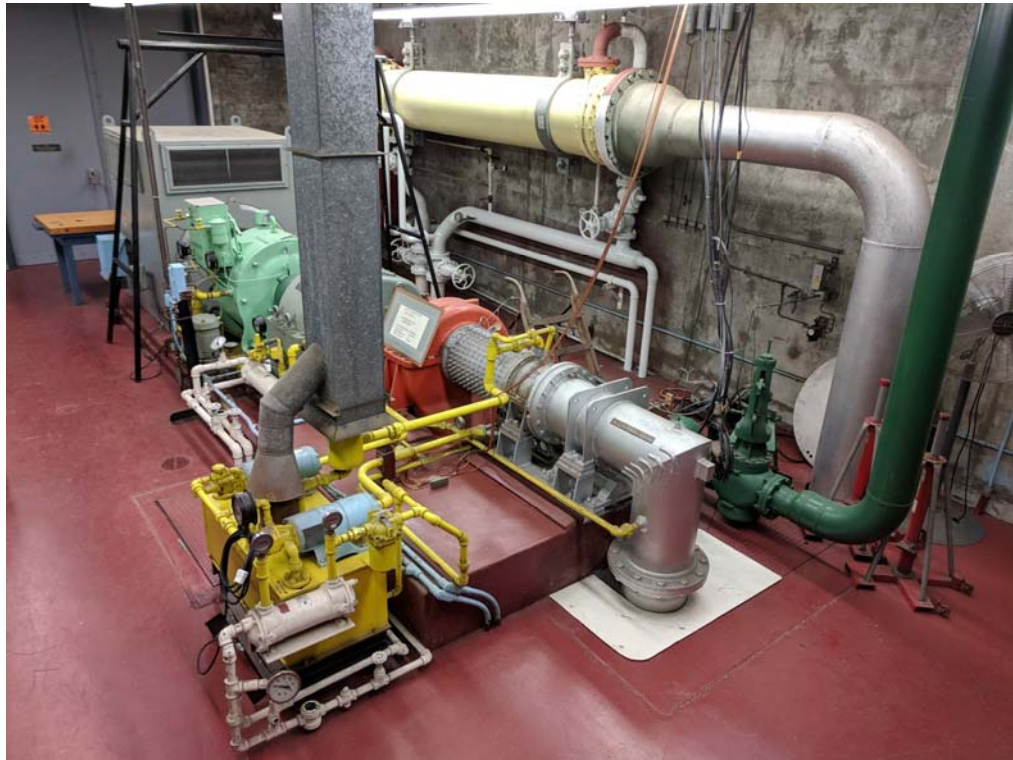
Figure 5. 1000 kW Allison Chamber Compressor
