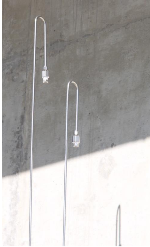
Figure 13. Vent Pipes Located Above Compression and Storage Station, with Mud Dauber Protective End Caps Installed, Turned Down to Prevent Rain Intrusion.
