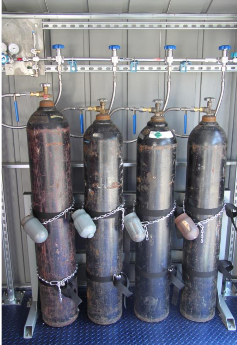
Figure 7. Four-cylinder Pressure Purge Station with Nitrogen Cylinders Connected, 34 atm (500 psig) Pressure Regulator, and Cross-purge Assembly.
