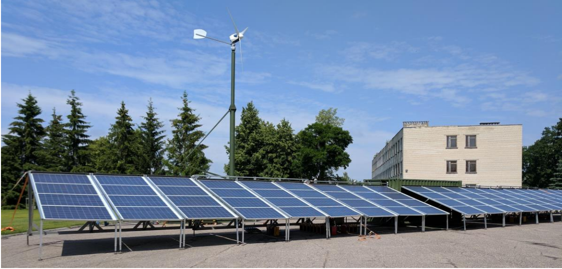
Figure 41. NATO Camp Hybrid Power Station
