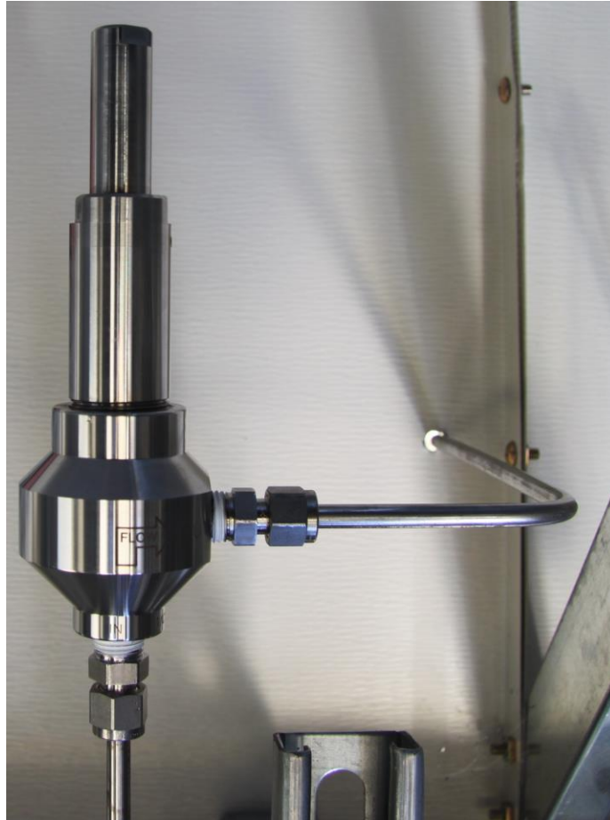
Figure 10. Proportional Safety Relief Valve Set to Operate at 34 Bar (500 psig).
