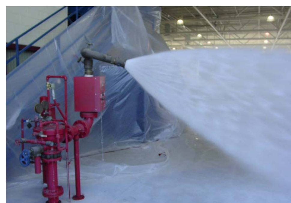
NoFoam System Nozzle Discharge Check at Arizona ANG, Tucson, AZ
