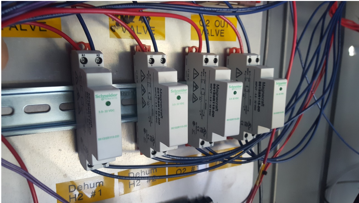
Figure 13. Magnecraft relays for control of dehumidifier power.
