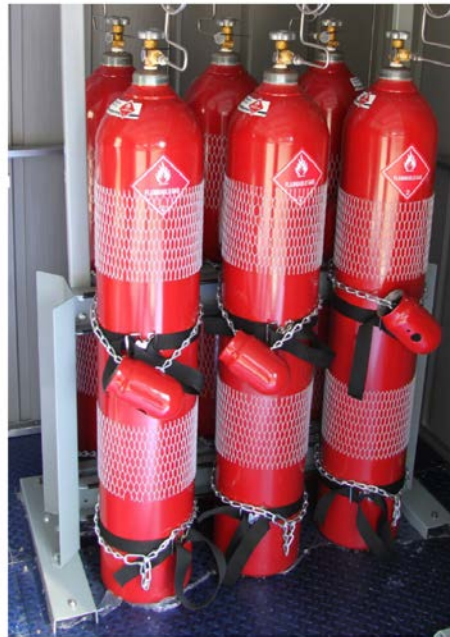
Figure 6. All-steel, standard size, compressed gas cylinders used for hydrogen storage
