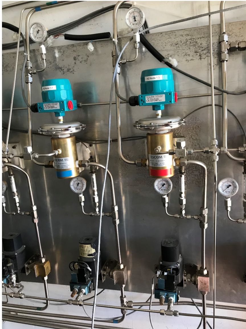
Figure 16. The hydrogen supply was outside the test cell and was piped into the cell through this system
