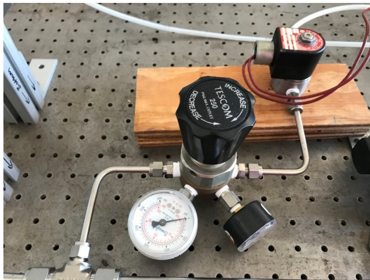
Figure 27. The cooling air pressure regulator and solenoid valve system
