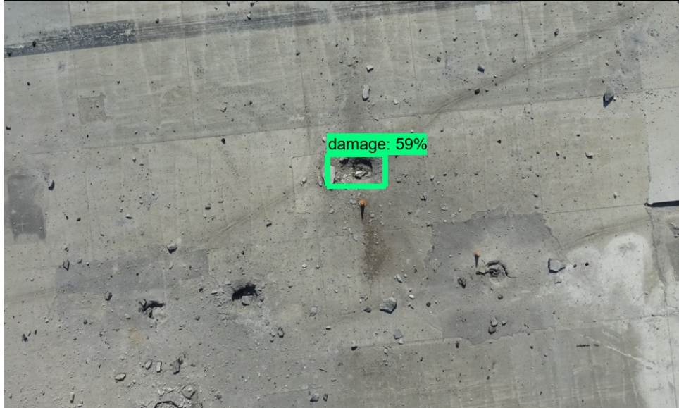
Figure 31. Single class damage detector model on airfield damage caused by explosives.
