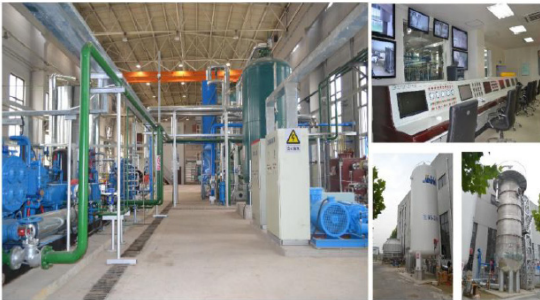
Figure 15. A 1.5 MW SC-CAES Plant in China. Source: [19].
