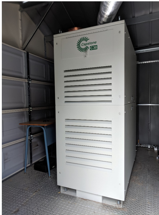
Figure 16. Low-pressure C30 inside the protective shed with the exhaust duct visible near the top of the image
