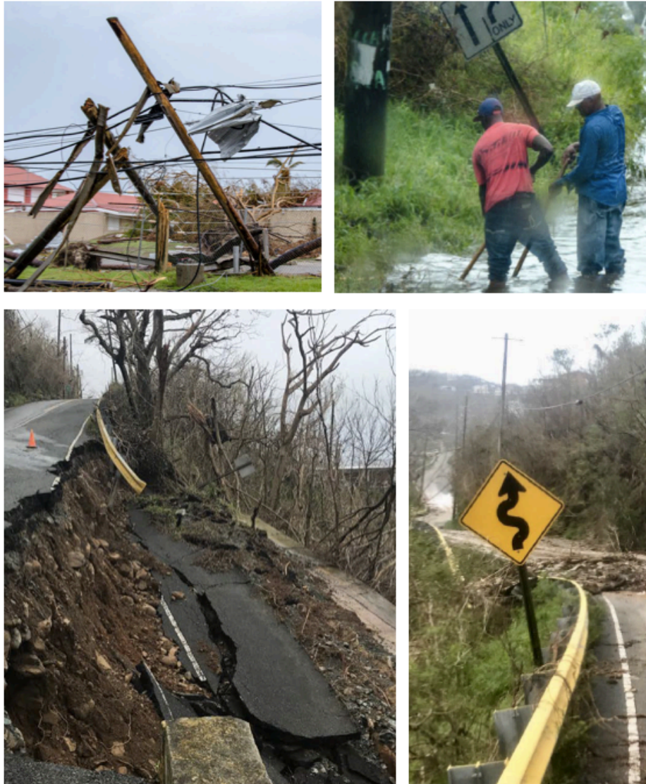
Figure 1.5. Examples of Damage to Critical Infrastructures in the USVI following Hurricanes Irma and Maria. Source: USVI Hurricane Recovery and Resilience Task Force (2018).
