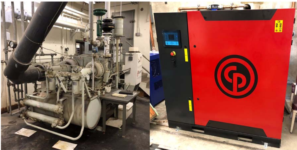
Figure 4. Legacy 500 kW Elliot Compressor Versus New 55 kW Chicago Pneumatic Compressor. Source: [1].
