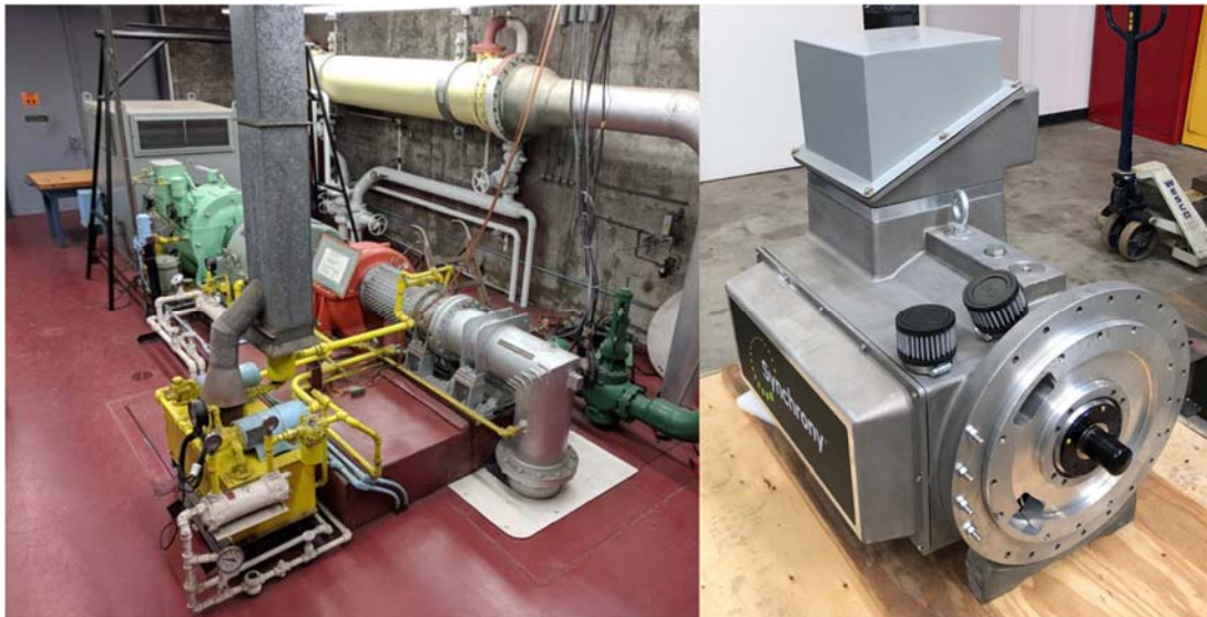
Figure 2. Legacy 1000 kW Allison-Chalmers Compressor Versus New 300 kW Synchrony Electric Motor. Source: [1].
