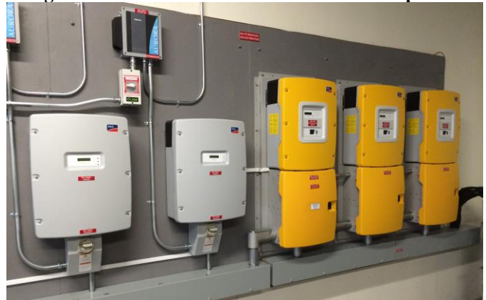
Figure 7. Installed 3 phase 208V microgrid.
