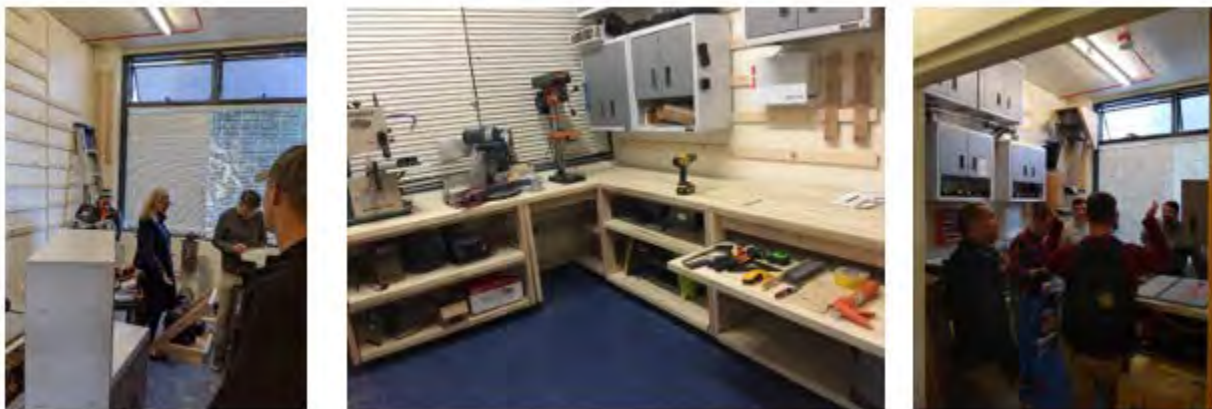
Figure 46. New shop: French Cleat installation ( left ), tools and drawers ( center ), and French Cleat utilization and air filtration ( right )
