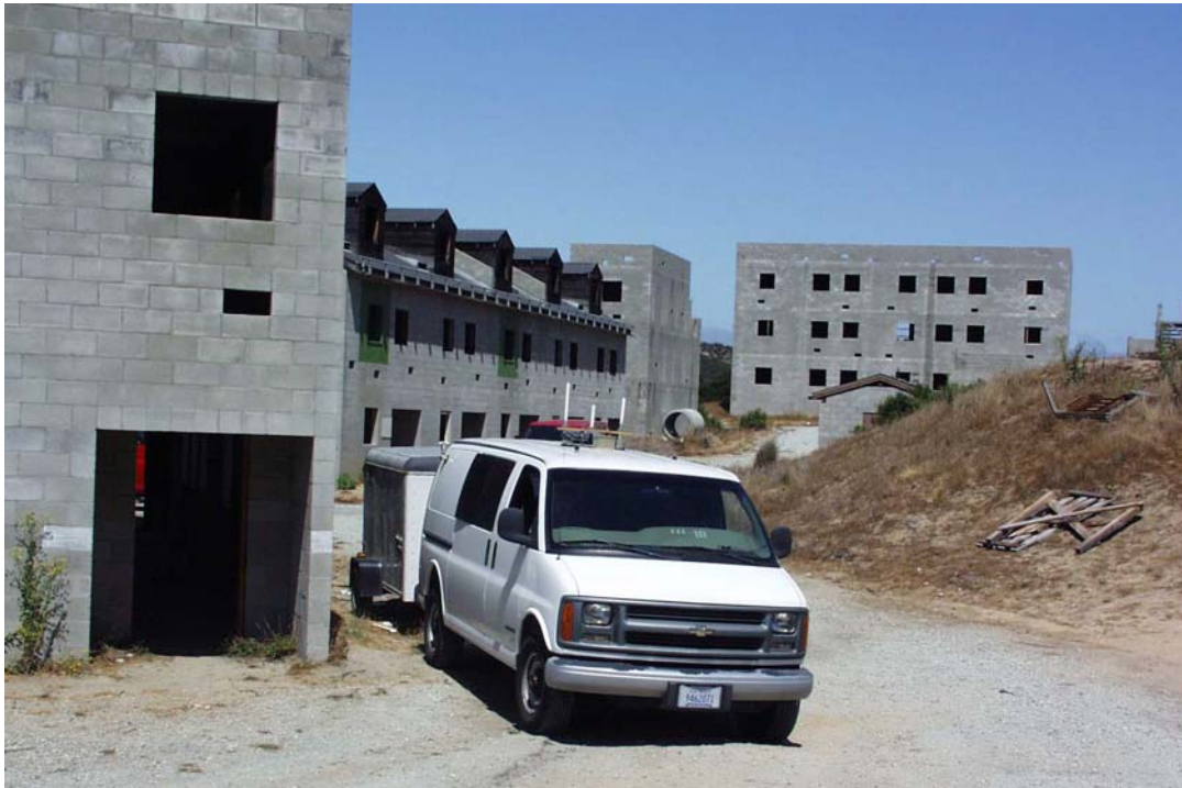
Figure 1 Photograph of Instrumentation Van at the MOUT Site
