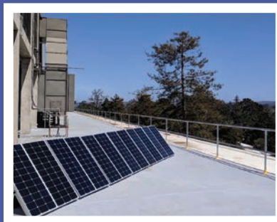
Setup of the PV panels at the Naval Postgraduate School.
