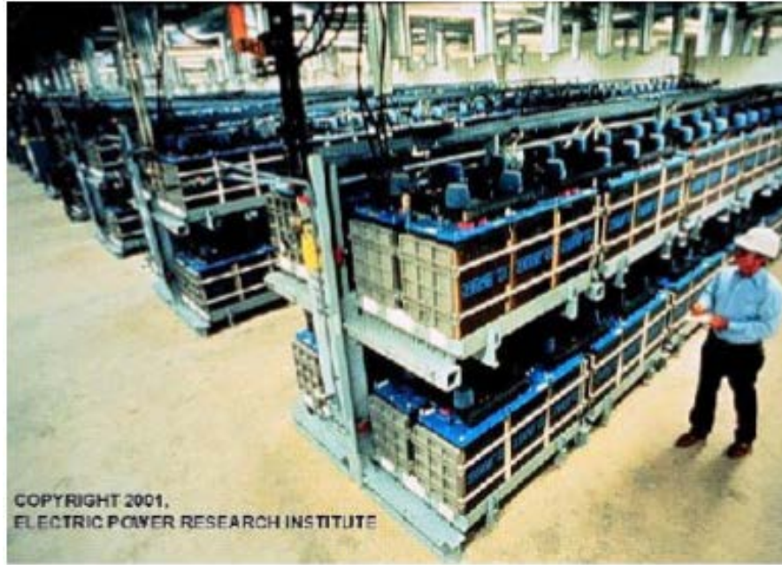
Figure 4. Example of a BESS. Source: Teleke (n.d.)
