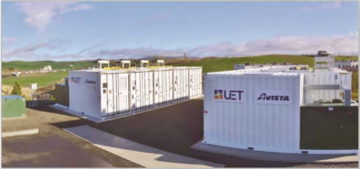
Figure 15. Uni.System installed at Schweltzer Engineering Laboratories in Pullman, Washington. Source: UniEnergy Technologies (n.d.-b).
